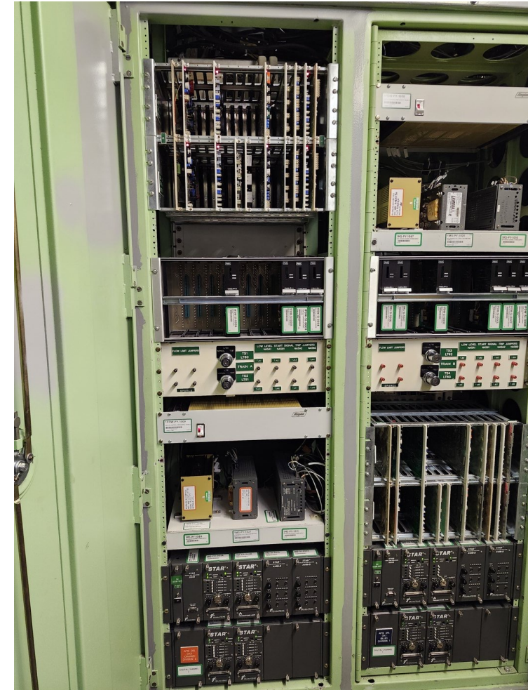
Original AFIS equipment — courtesy Duke Energy, INPO DI&C forum
