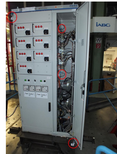
(Motor Control Center)
